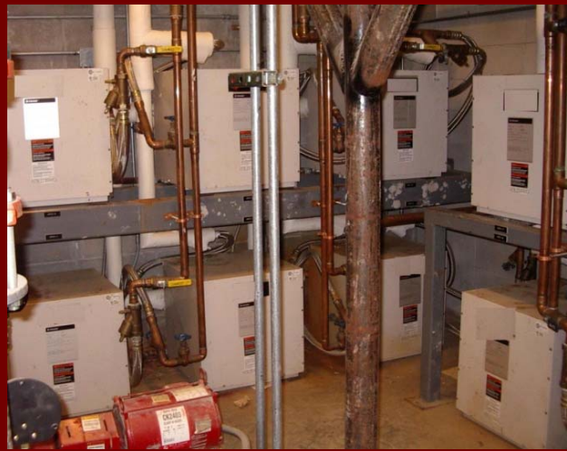
Water-to-Water Heat Pumps
