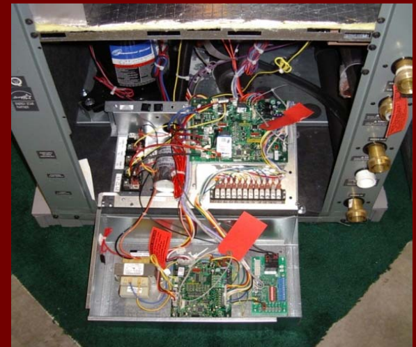
Hard to Service Heat Pumps
