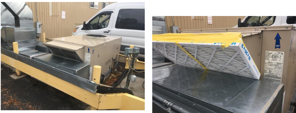
Figure 4. Picture of a MERV 13 filter installed on an outdoor air intake
